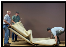
Grandfather and grandsons clearing out room to build dividing walls for an apartment.
